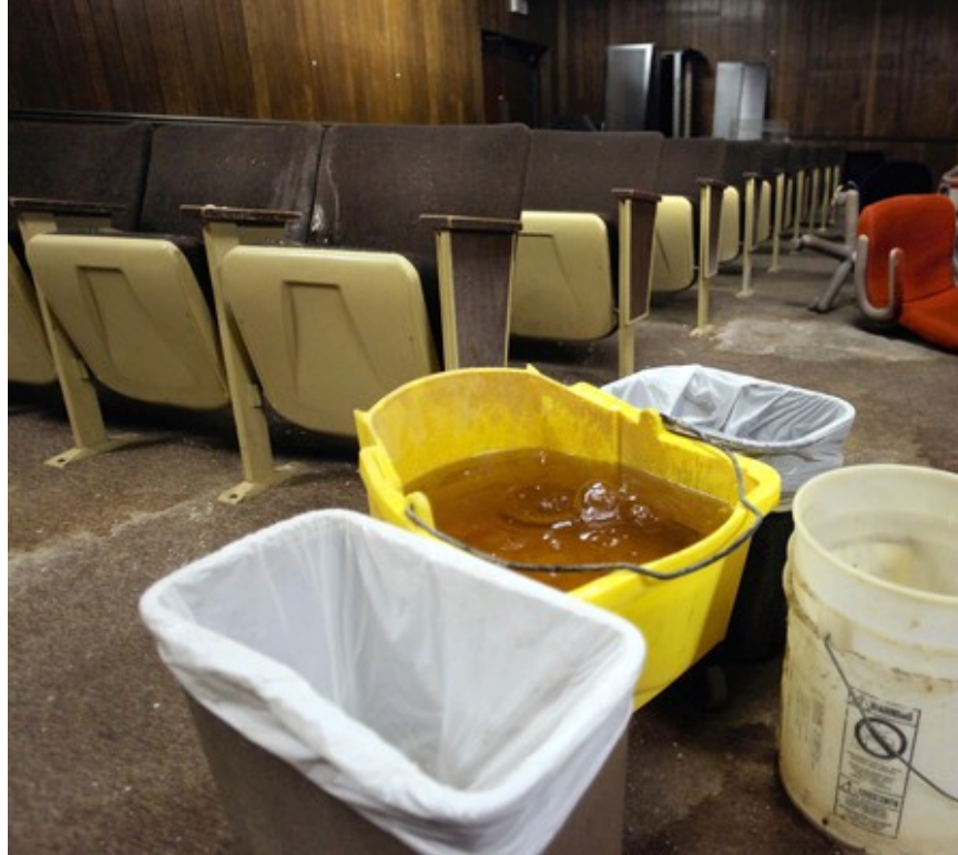
At the Franklin Park police station, water drips steadily from soggy ceiling tiles into plastic trash cans. (Chuck Berman, Chicago Tribune / March 7, 2011)
